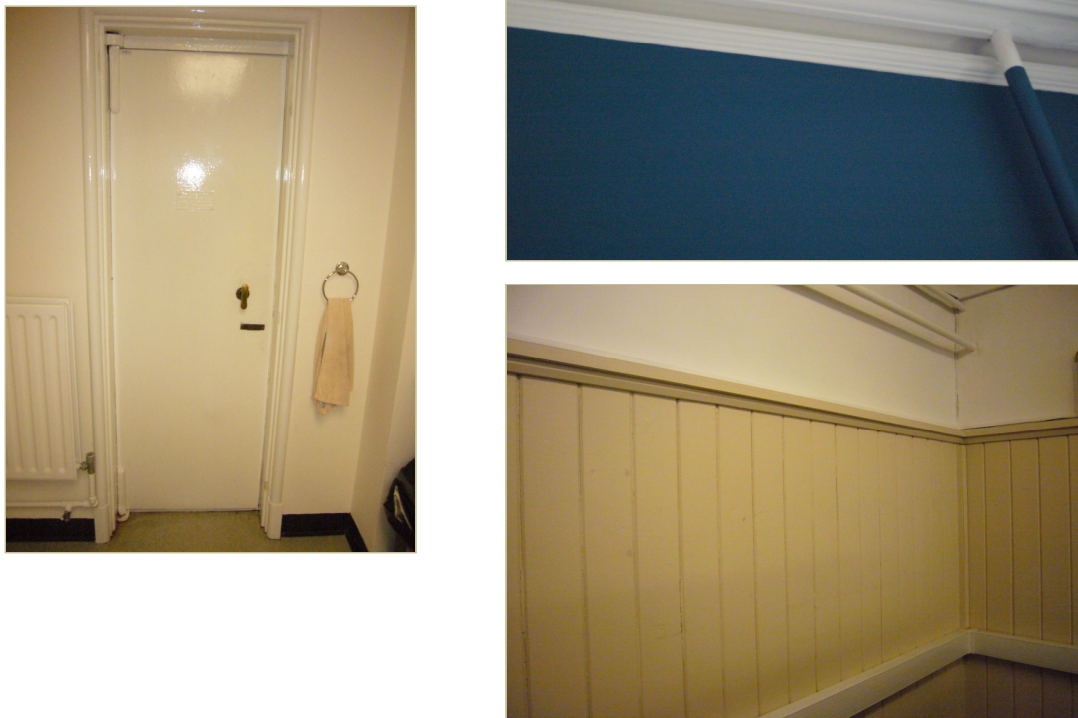
Figure 7. Left, original lift door in downstairs kitchen. Top Right, cornice moulding in Entrance Lobby. Bottom Right, wood panelling in Assistant Administrator's office in basement
