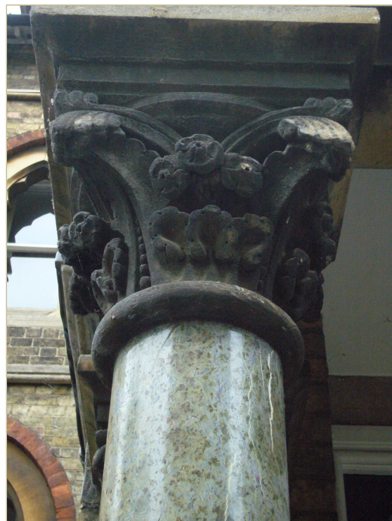
Figure 6. Blackening on the pillar capitals of the 1894 porch
