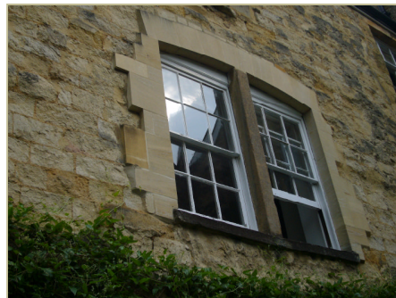
Figure 16. Left, repairs around the first-floor rear window. Top right, the St. Giles' frontage. Bottom right, repairs around the windows of the western wing
