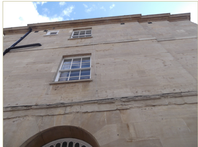
Figure 7. Damage to the façade and banding on the side (western) elevation
