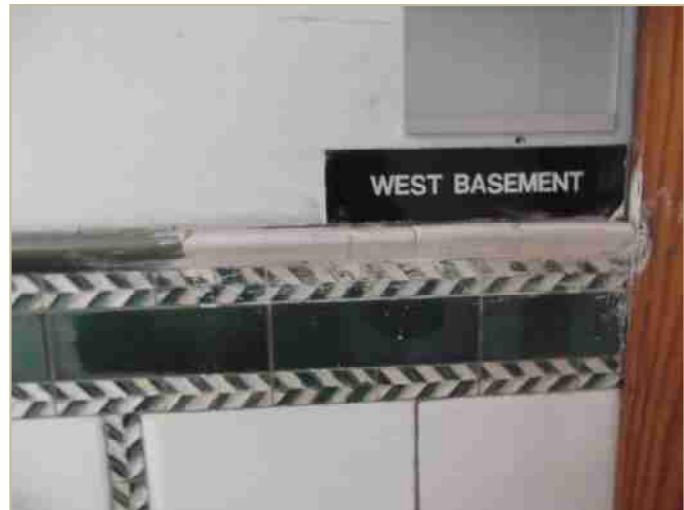
Figure 16. Unsympathetic repair to tiles on ground-floor corridor
